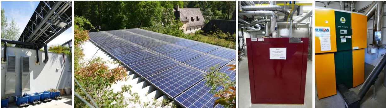
Solar thermal, photovoltaic, BHKW and wood chip heating in the zoo
