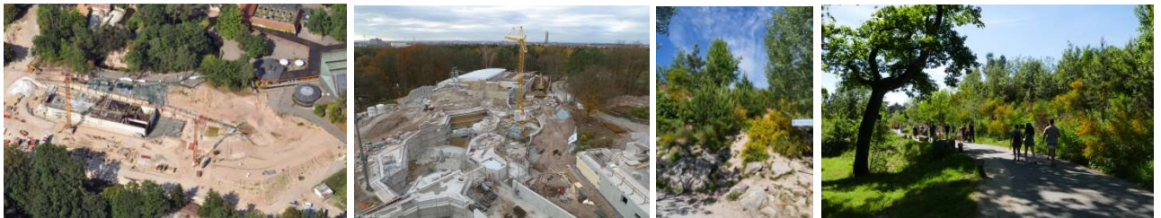
Of the 25,000 m 2 construction site for the lagoon, around 20,000 m 2 is now covered with vegetation.
