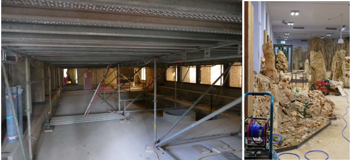
Small house - big change: The old hippo house during its metamorphosis into a desert house in February 2017 and January 2018. Verein der Tiergartenfreunde Nürnberg e.V. supported the project with 1,000,000 euros. Federal funding was about 200,000 euros.
